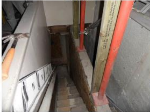
P9 – Propping on stairs (security screen at ground floor, first floor to be erected)
